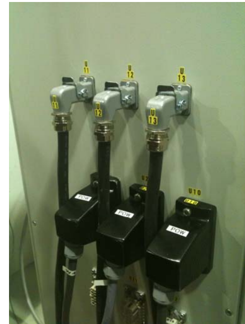
Prefixed cables between units
